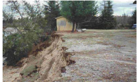
Eroding bank at the Cave-In
